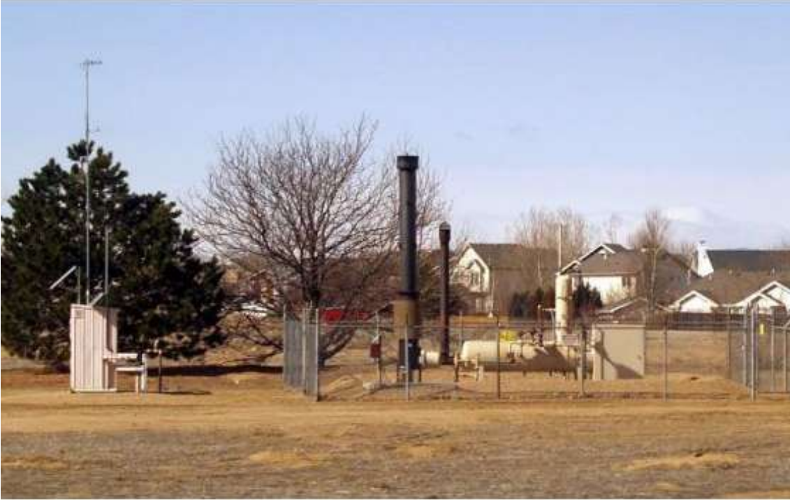
Figure 37. Greely Well in Subdivision 125
